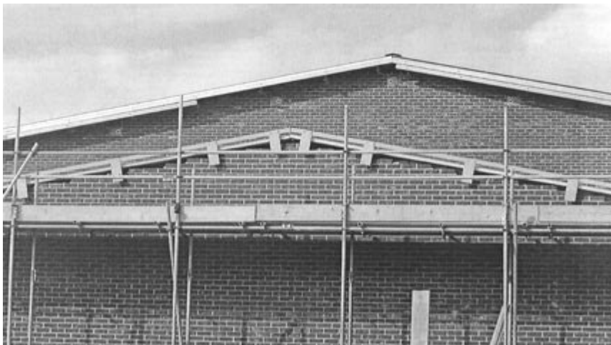
Figure 3 - Swift bricks under eaves
